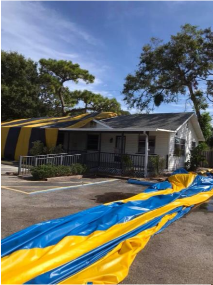
Tenting for termites (above) Volunteers cleaning up (right)
